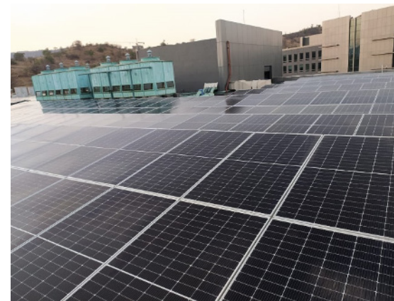
Installed Solar Photovoltaic Technology, Mono type, Pune Campus
